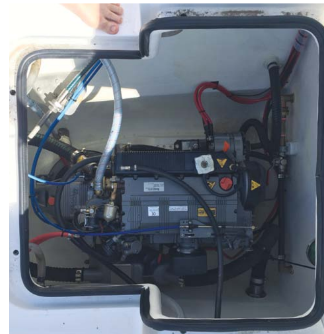
The standard Spirited 480 engine installation is outside of the accommodation area allowing for more space in the aft cabins and keeping the noise, smells and heat external.
